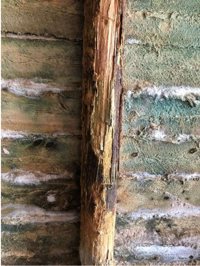
Photo 3: North Hampton – Wall and post rot
