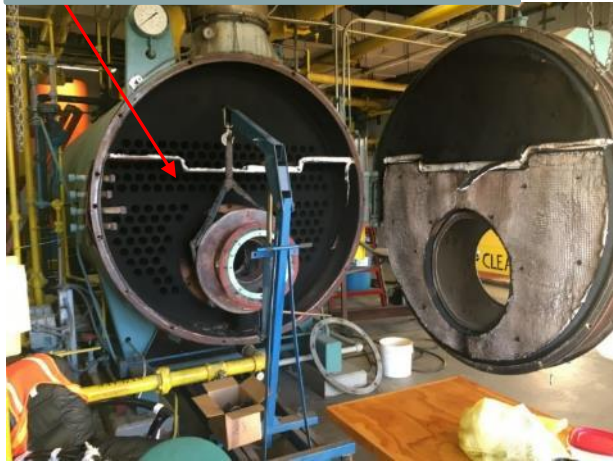
Steam tubes worn out
