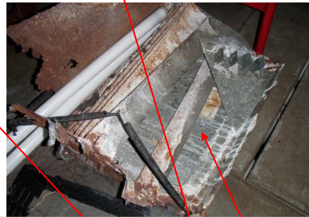
Duct work rusted through and collapsed
