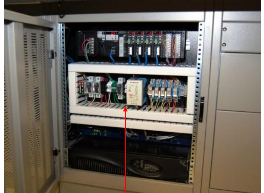
Old style door controllers
