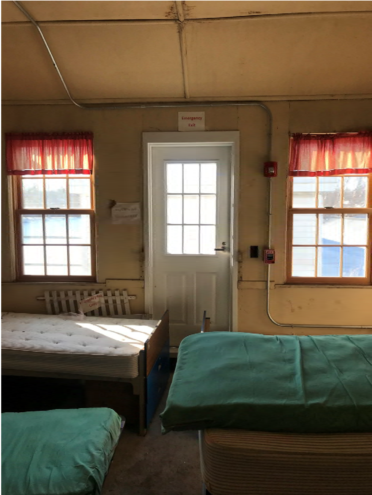
Figure 1 - Obstructed Door and Noncompliant Exit Sign
