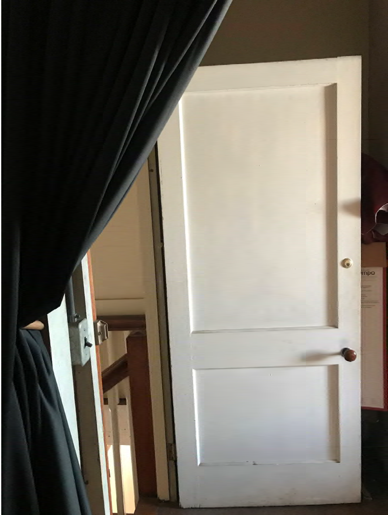
Figure 6 - Noncompliant door hardware and Unpermitted Dead Bolt
