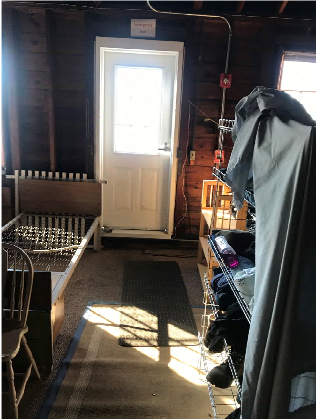
Figure 4 - Another Exit Door Obstructed and Noncompliant Exit Sign
