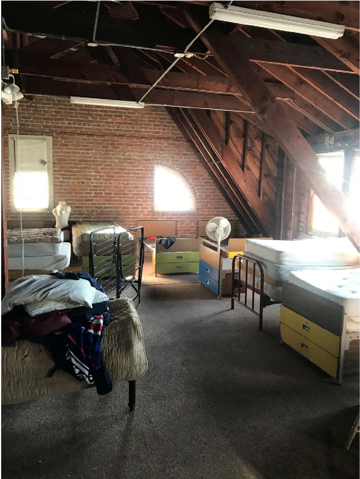
Figure 3 - Exit Aisles between Beds is Insufficient
