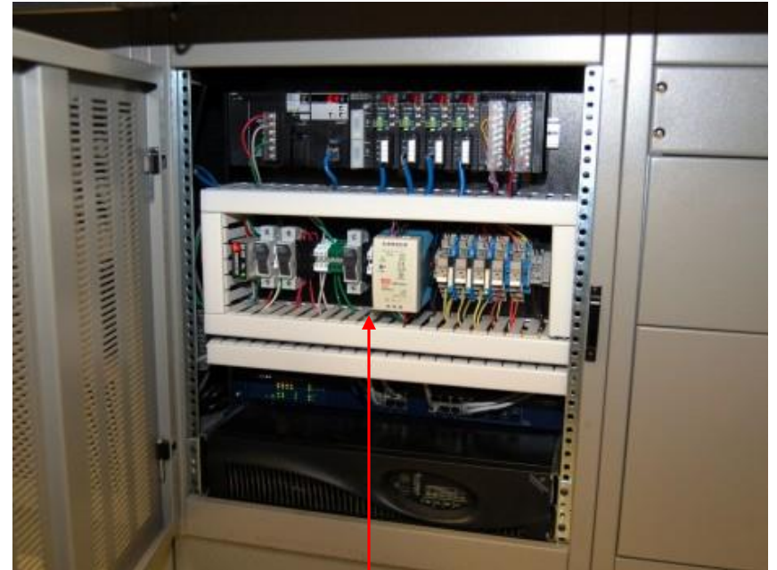
Old style door controllers
