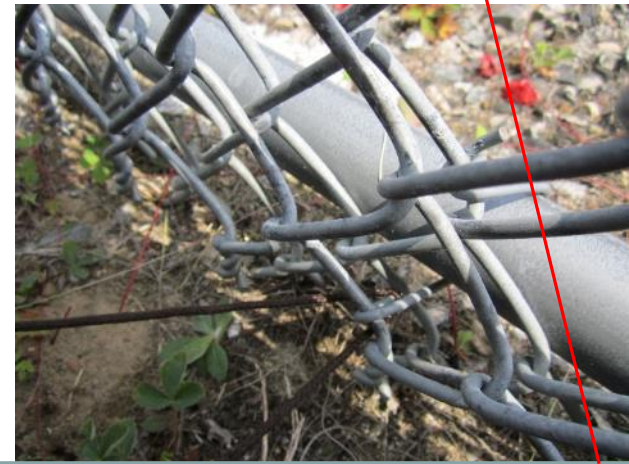
Old controllers exposed to elements
