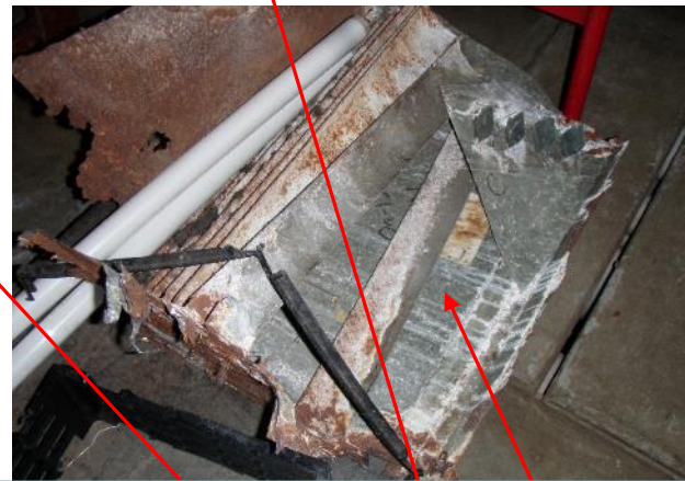
Duct work rusted through and collapsed
