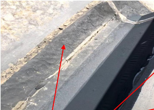
Cracks & sun damage in roof
