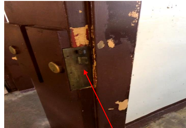
Door mechanisms worn out
