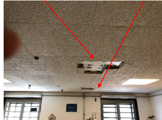
Ceiling falling down
