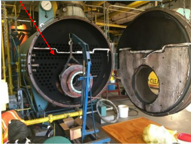
Steam tubes worn out
