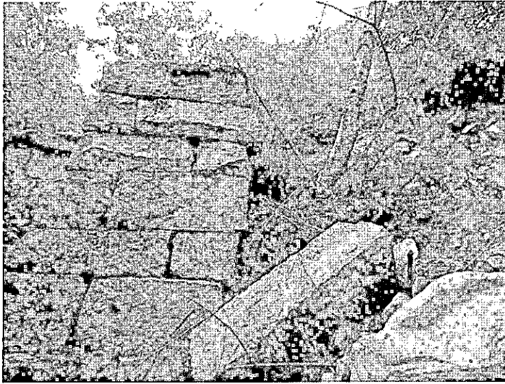
Mtn. Division Railroad Corridor, Harts Location Bridge #81.82 Failing N.E. Wing Slope
