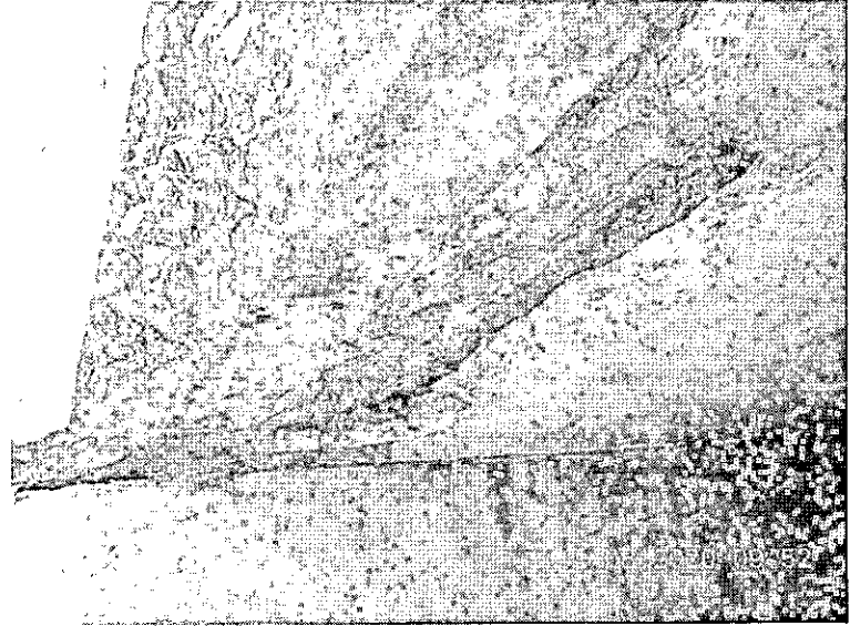
Concord-Lincoln Corridor, Tilton MP C19.66 Box Culvert Deterioration
