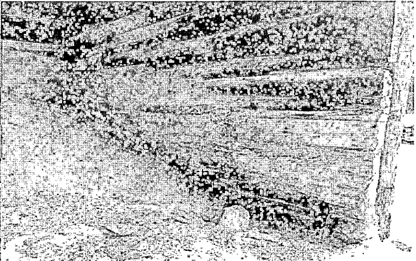
Belmont (314) – Deteriorated wall condition
