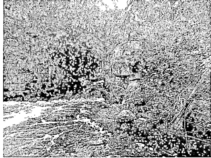
Concord-Lincoln Corridor, Concord Bridge #C5.20 Failing S.E. Dry Laid Stone Wing
