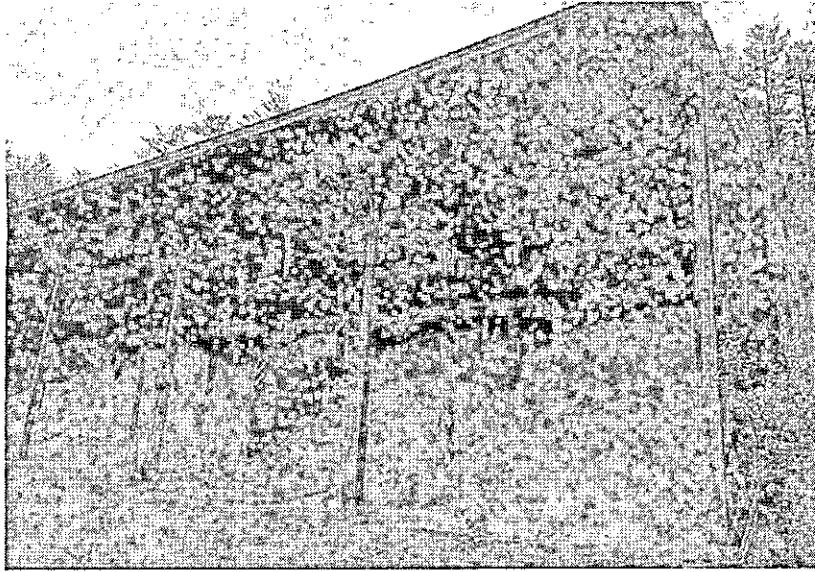
Warner (526) – Salt Shed inadequate capacity
