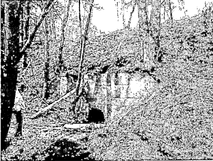
Concord-Lincoln Corridor, Canterbury Culvert MP C7.22 Vegetation Removal Required to Preserve Culvert Pipe Headwall Slope Retaining Structure
