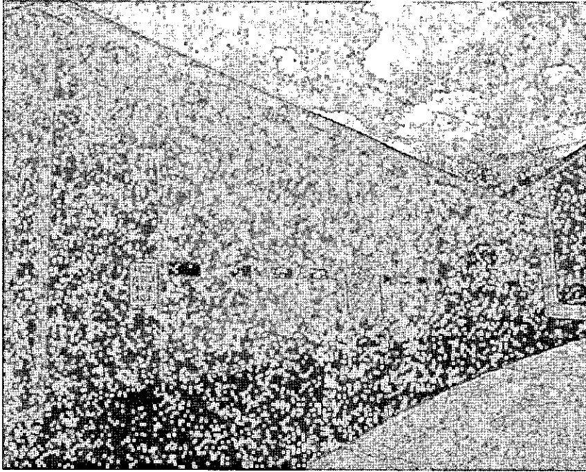
Front view of existing patrol shed. Garage doors need replacement and are undersized to safely accommodate the vehicles and equipment.
