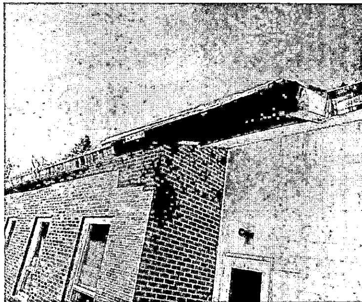
Close-up view of the holes in the trim and soffit where pigeons and animals gain access to the interior of the building.
