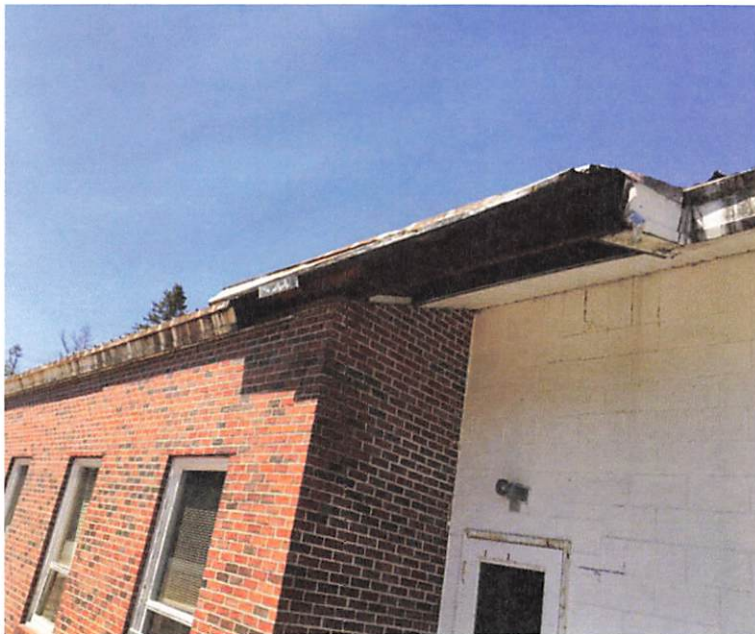
Close-up view of the holes in the trim and soffit where pigeons and animals gain access to the interior of the building.
