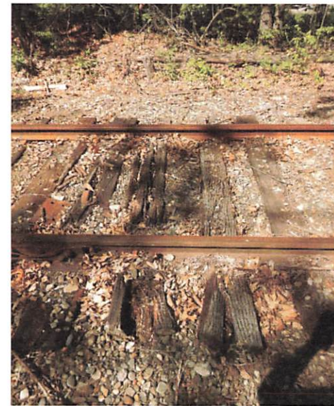
Concord-Lincoln Corridor, Concord Timber Railroad Ties
