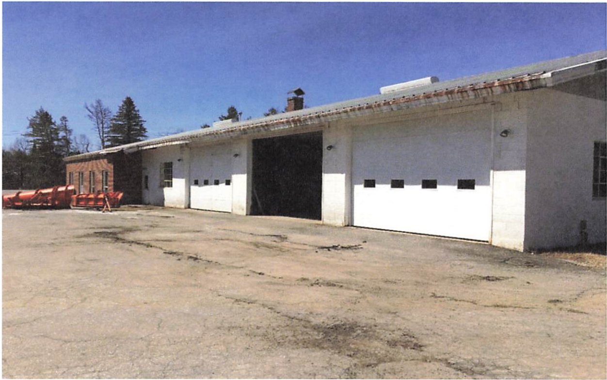
Rear right side view of existing building. Siding and building trim in need of replacement. Note holes in roof trim where pigeons and animals have access to shed interior. Also, shed end of roof is too low for building extension to increase storage or headroom inside the building.
