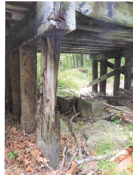
Concord-Lincoln Corridor, Woodstock Bridge #P18.17 Deteriorated Timber Bent Post
