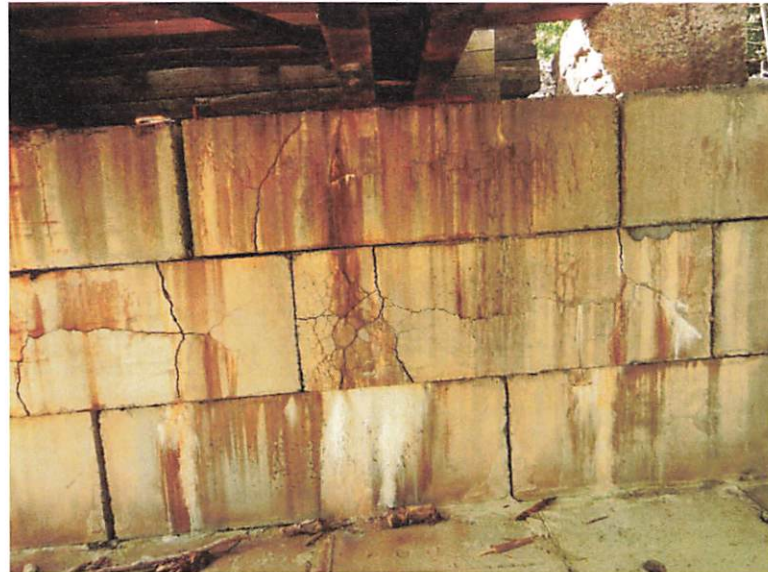
Mtn. Division Railroad Corridor, Harts Location Bridge #82.96 Failing East Abutment
