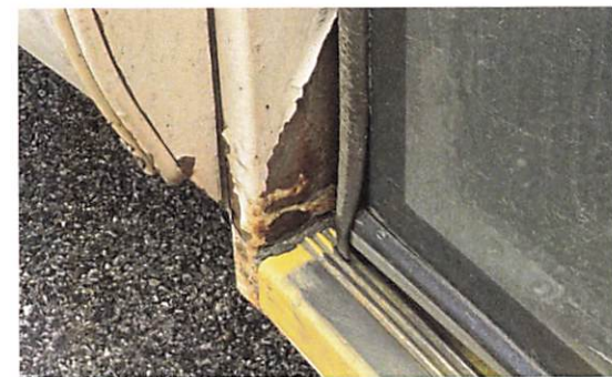
VNA@HCS: Corrosion affecting passenger door
