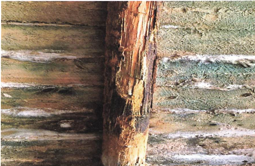
North Hampton (612) – Wall and post rot
