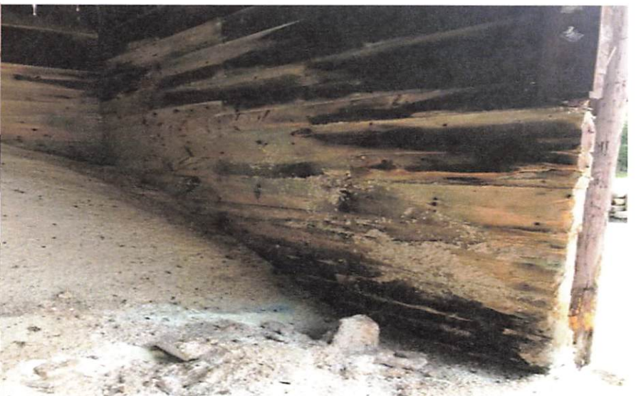
Belmont (314) – Deteriorated wall condition
