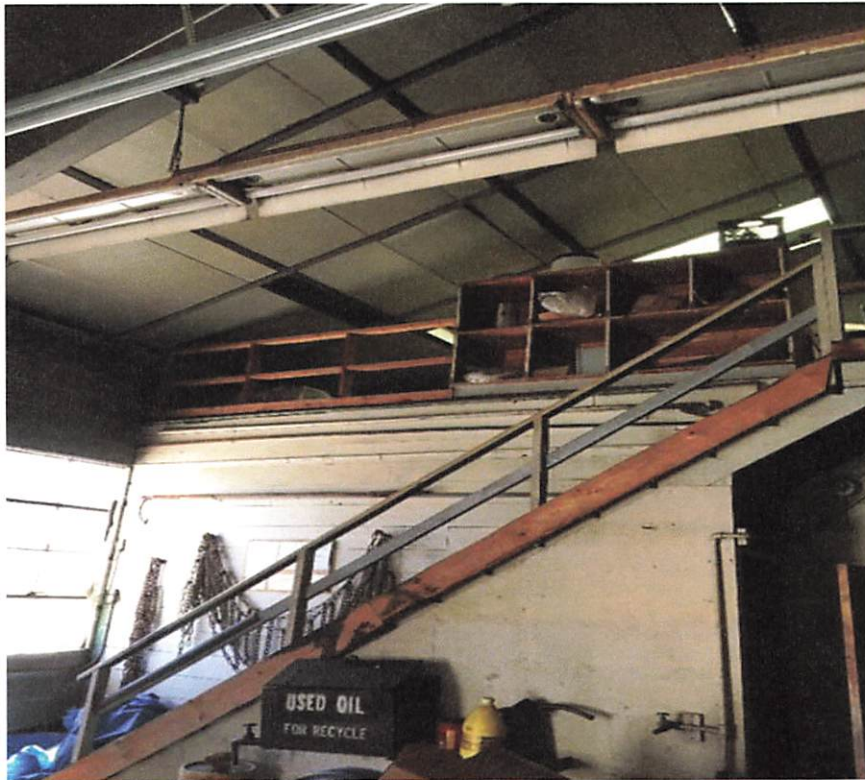
View of interior of building. Note uninsulated ceiling panels.
