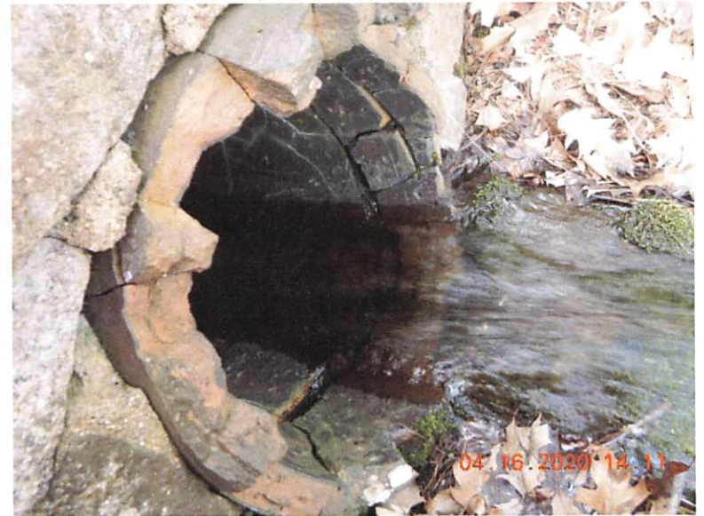
Concord-Lincoln Corridor, Laconia MP C34.91 Pipe Failure
