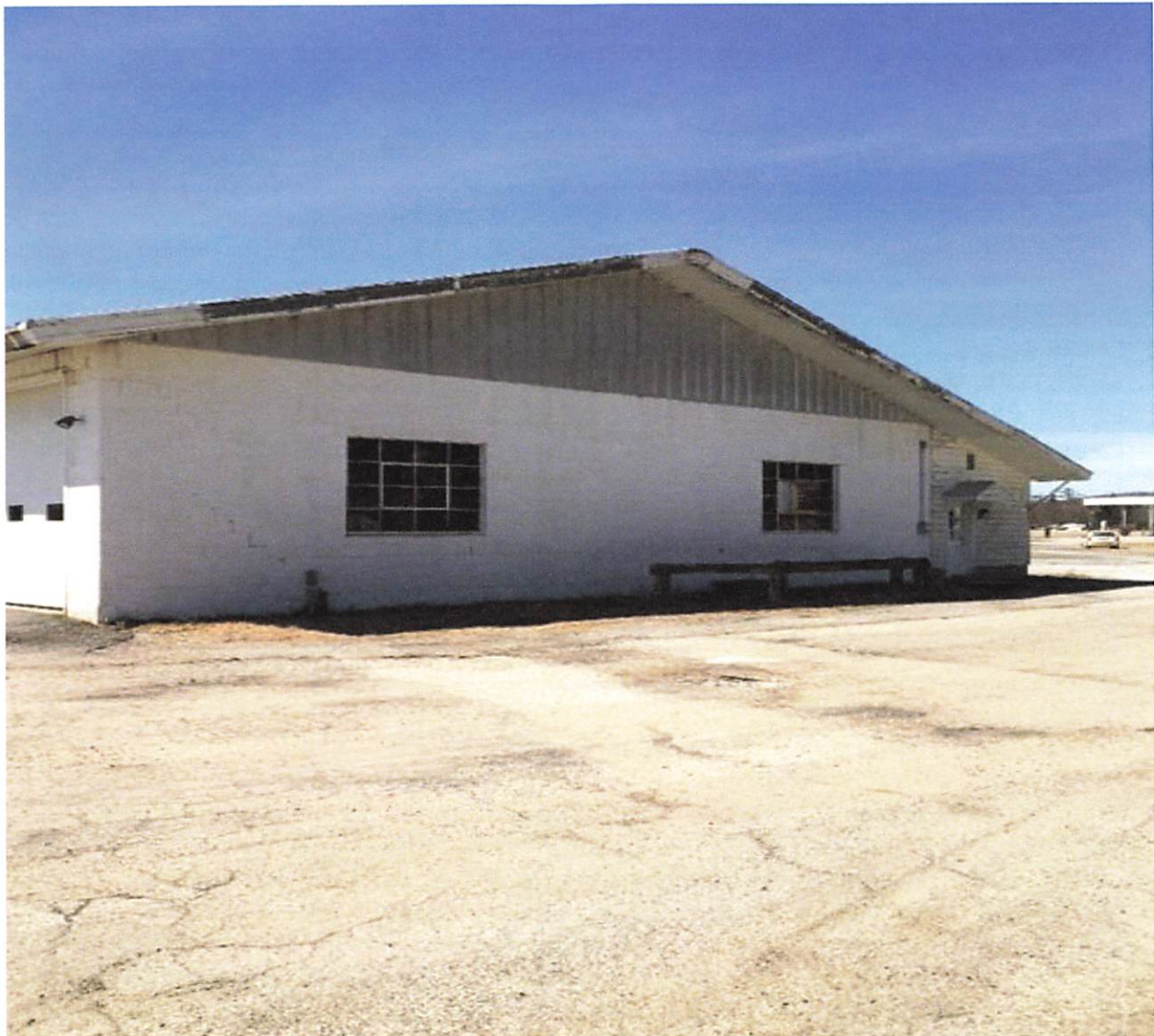
Rear view of existing building. Note deteriorated condition, single pane windows, rotten trim and cracks in uninsulated cinder block walls.
