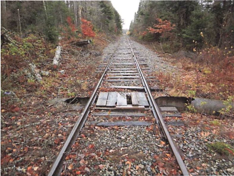
Mt. Division Railroad Corridor, Carroll MP 95.21 Culvert Pipe Failure
