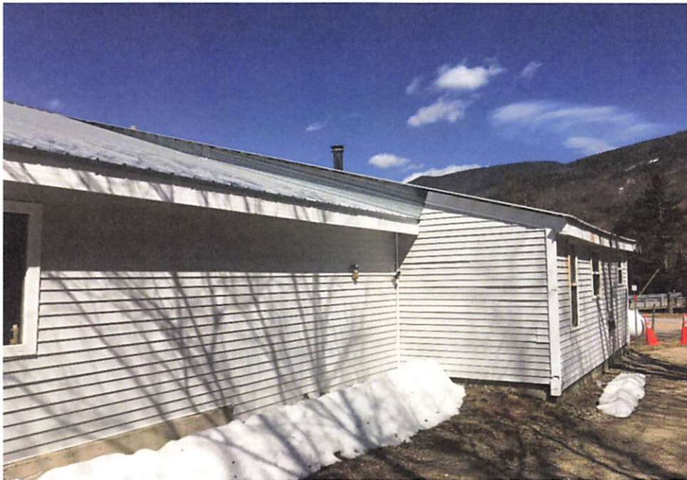
Rear view of existing patrol shed. Siding and building trim in need of replacement. Shed end of roof is too low for building extension to increase storage or headroom inside the building.
