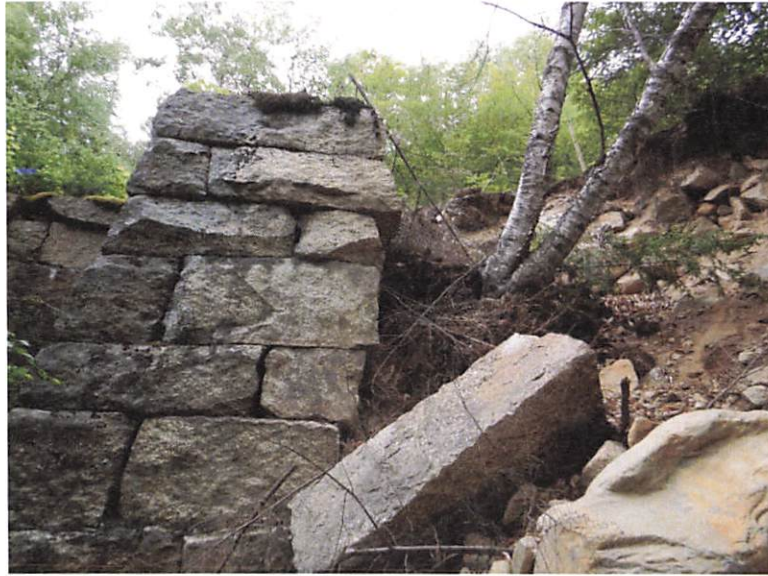
Mtn. Division Railroad Corridor, Harts Location Bridge #81.82 Failing N.E. Wing Slope
